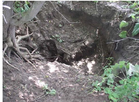
Sinkhole in the UIRW.
